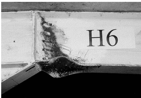
Fig. 4 View after failure of H6
