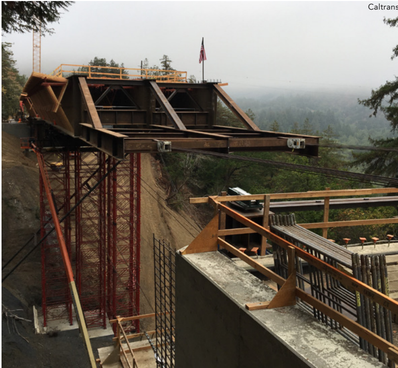
Pfeiffer Canyon Bridge, Big Sur, Calif. 2020 Prize Bridge Merit Award – Long Span
