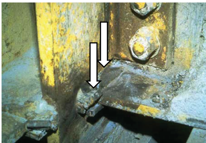
Fig. 6-2. Fracture of beam flange at CJP groove weld of beam flange to column flange. (Photo by Dave Norris)
