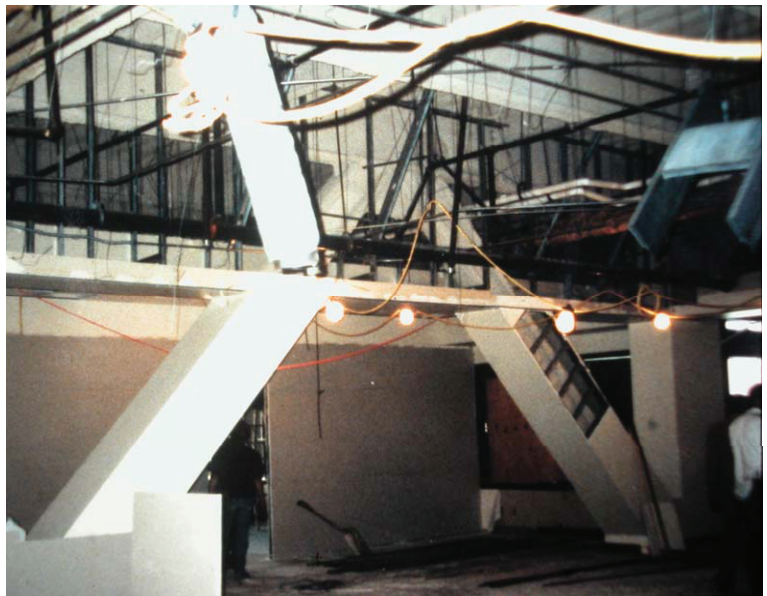
Fig. 10-8. Buckled chevron-pattern brace at the California Federal Savings data processing center. (Photo courtesy of P. Yanev)
