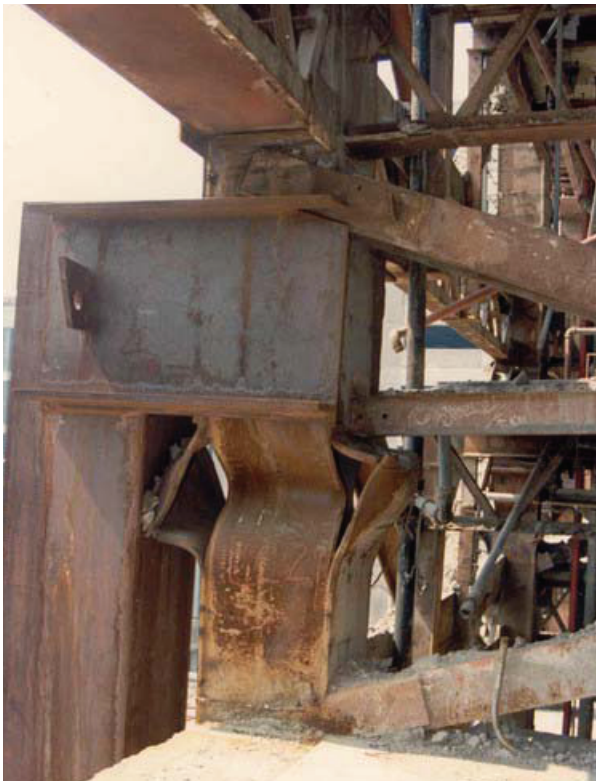
Fig. 10-7. Failed built-up box column in one of the surviving Piño Suarez Towers. (Photo courtesy of John Osteraas)
