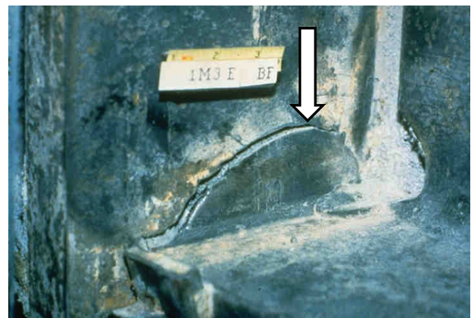
Fig. 6-3. Fracture involving divot of steel being withdrawn from column flange. (Photo by Dave Norris)
