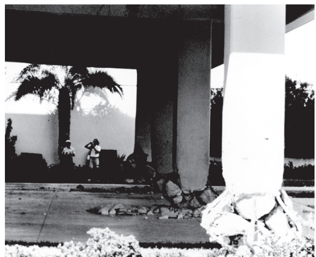
Fig. 10-6. Crushed columns at base of Imperial County Services Building. (Photo courtesy of U.S. Geologic Survey)
