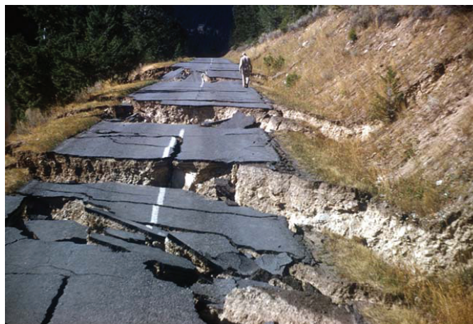
Fig. 1-9. Lateral spreading damage to highway pavement near Yellowstone Park, 1959 Hebgen Lake earthquake. (Photo courtesy of U.S. Geologic Survey)
