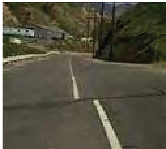
Fig. 1-7. Offset of highway centerline, 1988 Spitak, Armenia, earthquake. (Photo by P. Yanev)
