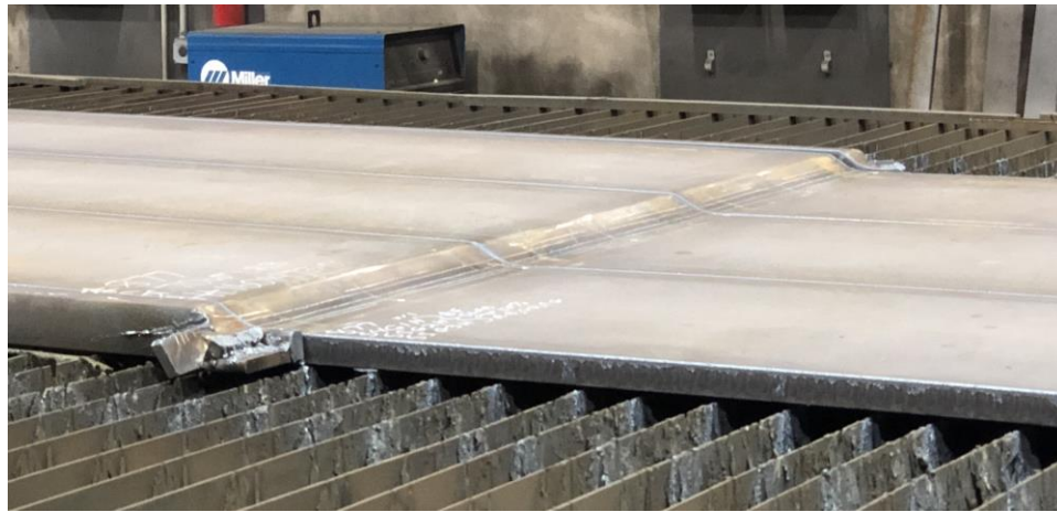
Figure 7 Photo in a fabrication shop showing the butt welding of steel plate slabs prior to cutting the flanges
