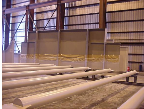
Figure 18 Photo showing painted members in a fabrication shop, note the masked area is for prime coat only
