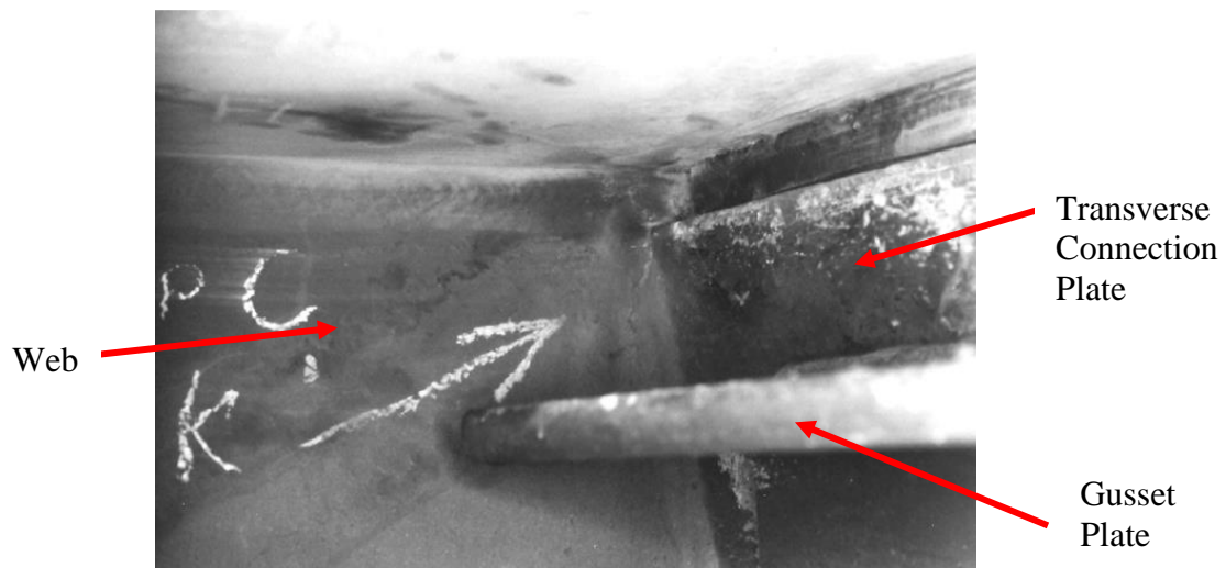
Figure 17 Web Cracking at Box Girder Diaphragm Connection Plate
