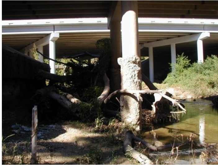
Figure 9 A drilled shaft that has experienced severe scour.
