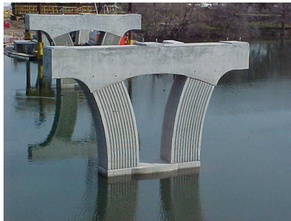
Figure 19 Multi-column piers with haunched pier caps and curved columns with formliner treatments.
