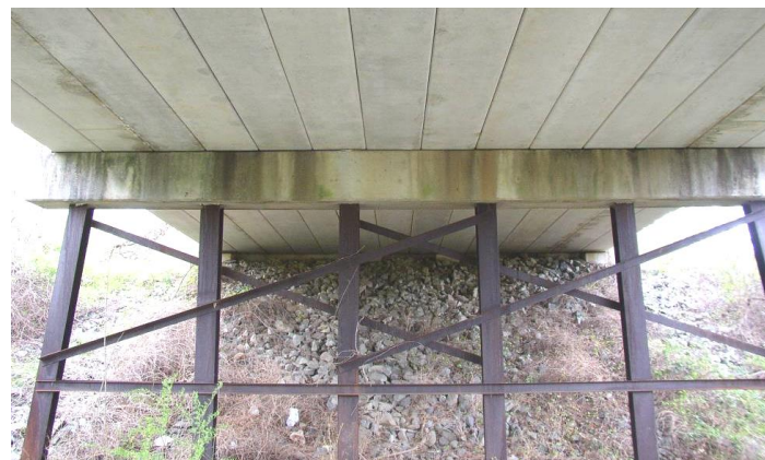
Figure 23 Pile bent with braced steel H-piles serving as both columns and foundations.
