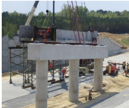
Figure 18 Typical pier with round columns and a prismatic pier cap with individual pedestals for each bearing.
