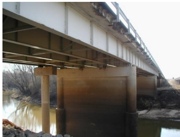
Figure 31 Multi-column piers with web walls, and single column hammerhead piers supporting a later widening.
