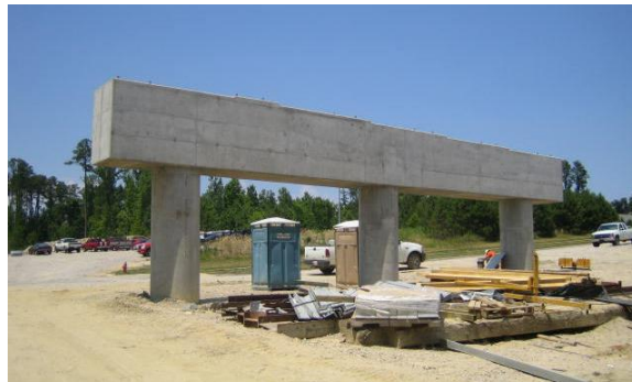
Figure 17 Typical pier with round columns and a pier cap stepped at each bearing.
