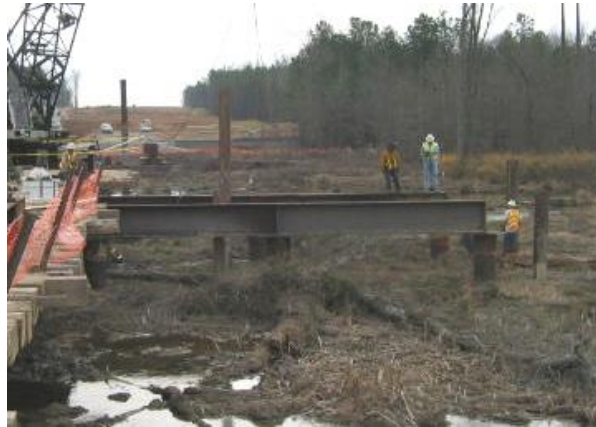
Figure 27 Temporary work bridge with steel pipe piles, steel pier caps, and a timber deck.
