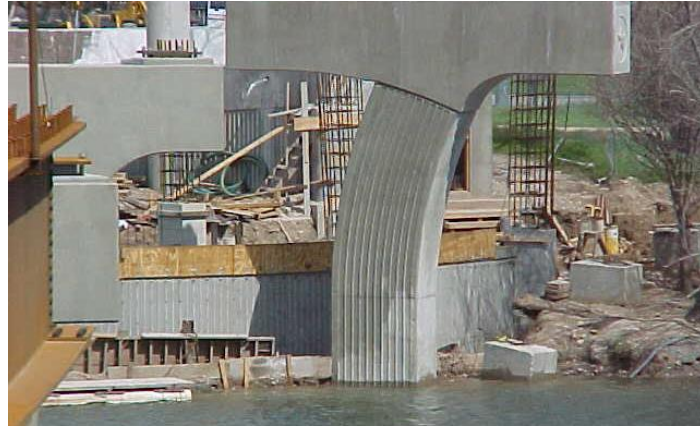
Figure 22 Single column piers with haunched pier caps and single, unsymmetrical curved columns with form liner treatments.
