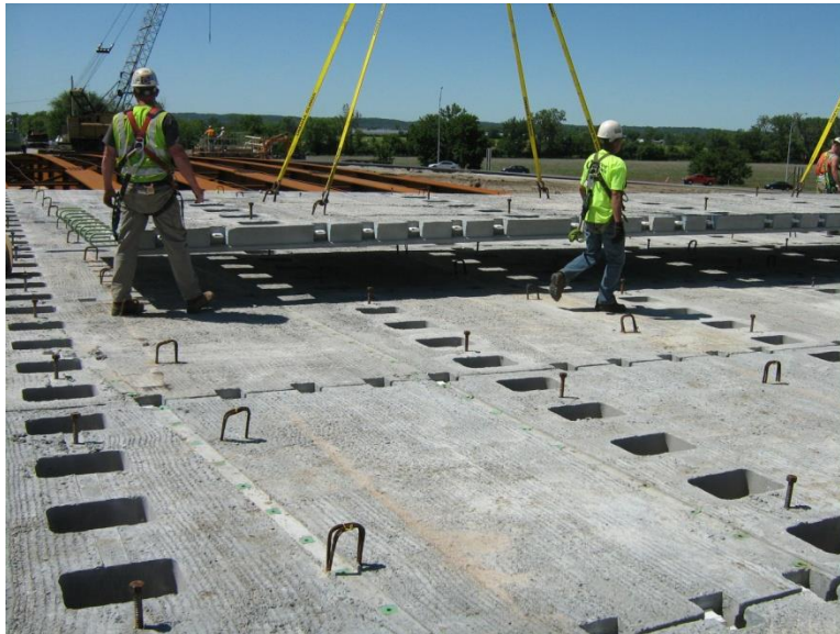
Figure 1 Bridge deck being constructed with full depth precast concrete deck panels (courtesy Iowa DOT).
