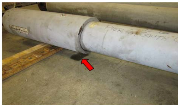
Figure 17: Existing Leaking STU
