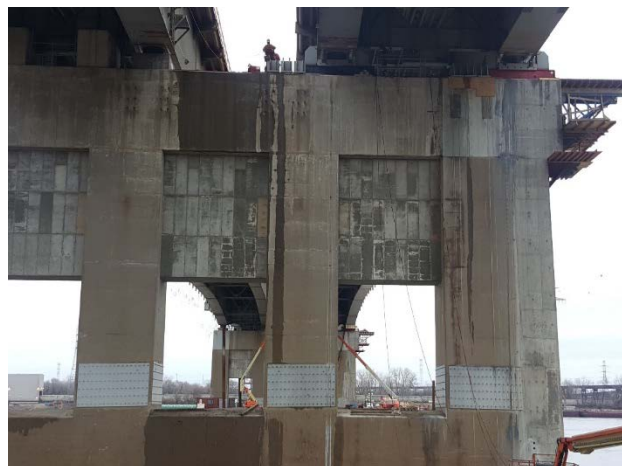
Figure 9: Post-Slide at Pier 2
