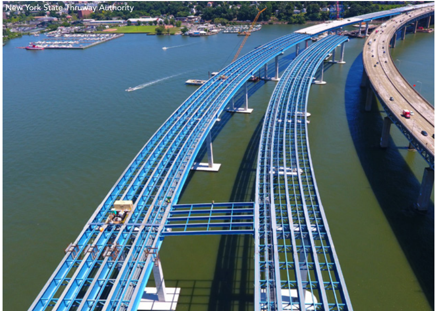
Governor Mario M. Cuomo Bridge Westchester/Rockland Counties, N.Y. 2020 Prize Bridge National Award – Major Span
