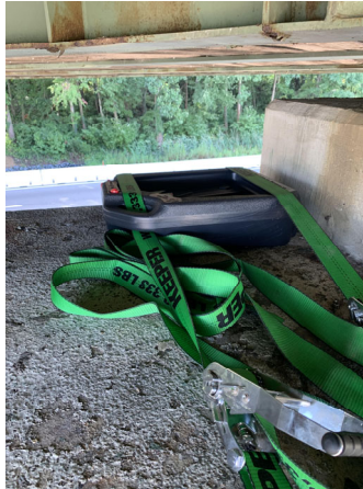
Figure 3-9. Water Collection on the Chapman Rd. Bridge
