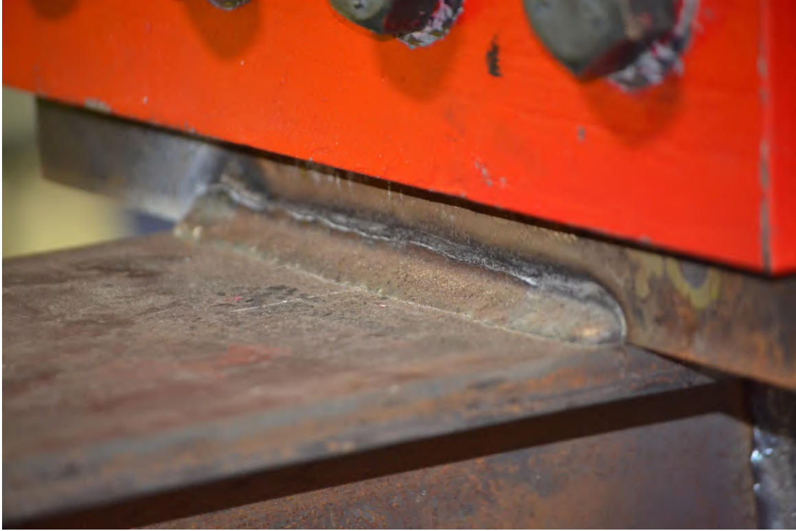
Figure A-149: Weld condition of W10X39-ST-E4 after testing (Side 1)
