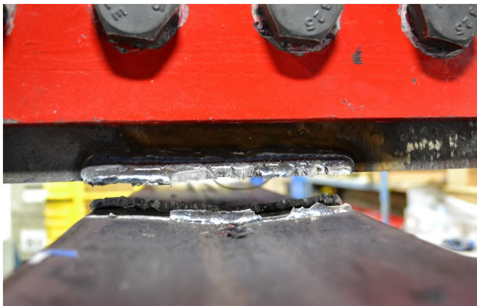
Figure 3.7-30: Weld fracture of W12X26-ST-NA
