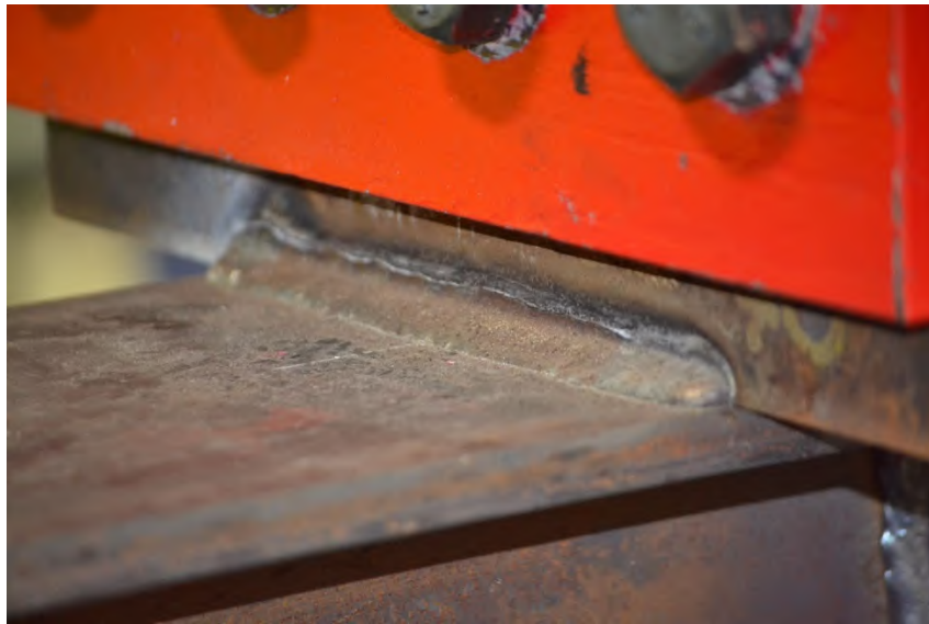
Figure 3.7-33: Weld condition of W10X39-ST-E4 after testing (Side 1)
