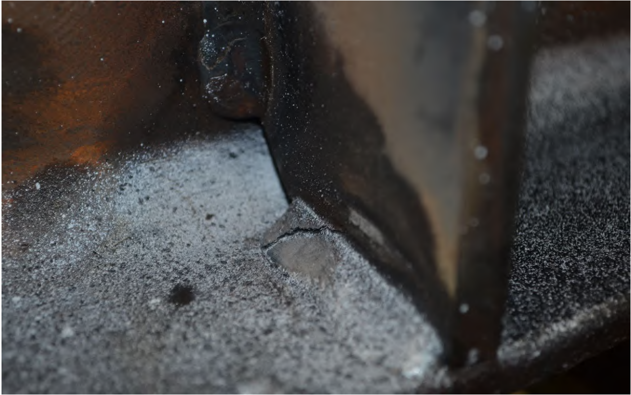
Figure A-82: Bottom flange to stiffener weld condition after testing
