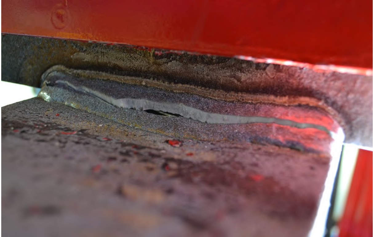
Figure A-136: Weld fracture of W16X31-ST-E3 after testing (Side 1)
