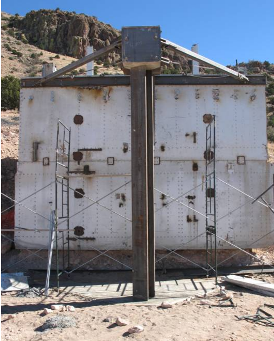
Figure 2-6. Photographs of the of the test article during curing of the footing.
