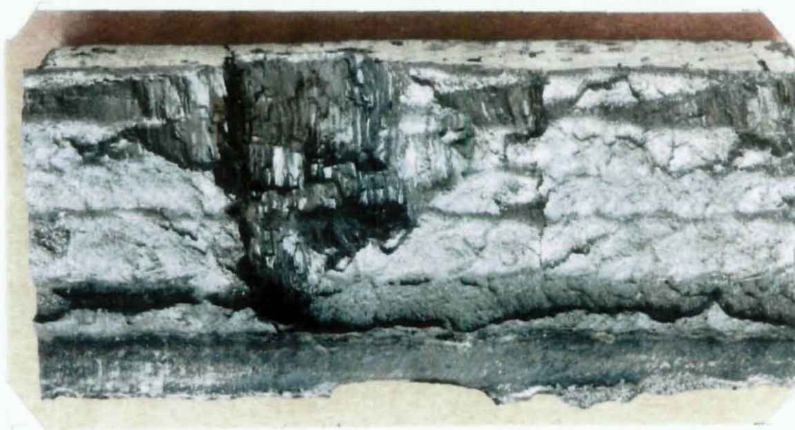
Figure 22. Center piece from the beam-side fracture of the east-beam top-flange joint.
