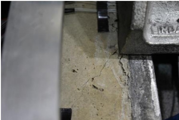
Unusual concrete crack adjacent to Clamp 1
