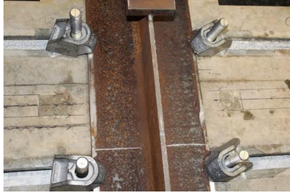
Abrasion on the steel flanges
