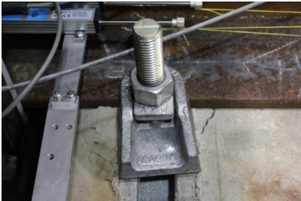
Concrete crack adjacent to Clamp 1
