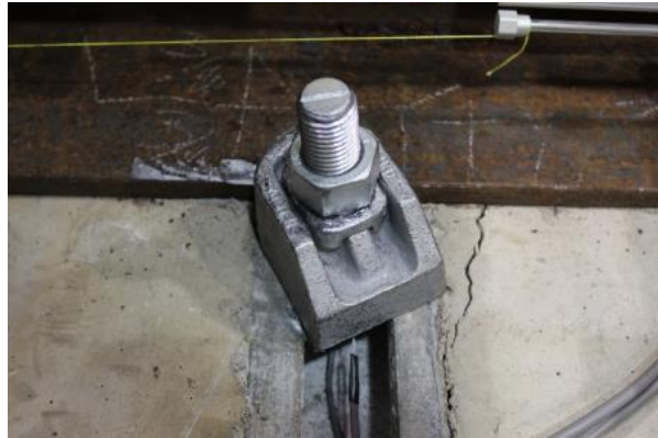
Concrete crack adjacent to clamp 1
