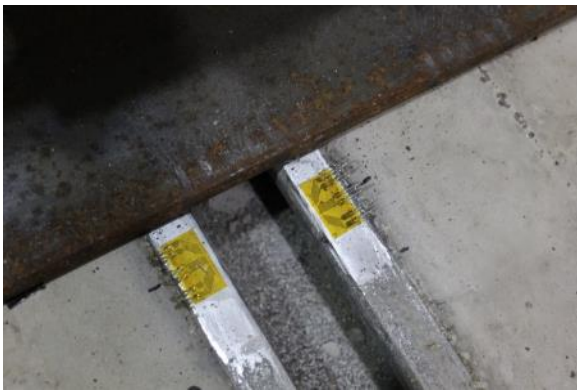
(1) Channel lip deformation
