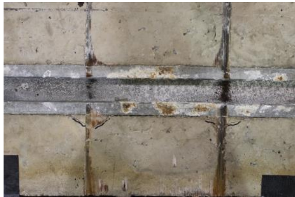
Cracks in the vicinity of the bolts
