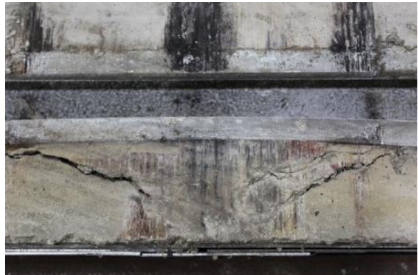
Concrete crack and bent channel lips adjacent to rear clamps
