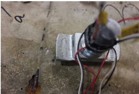
(3) Cracking in the bolt head
