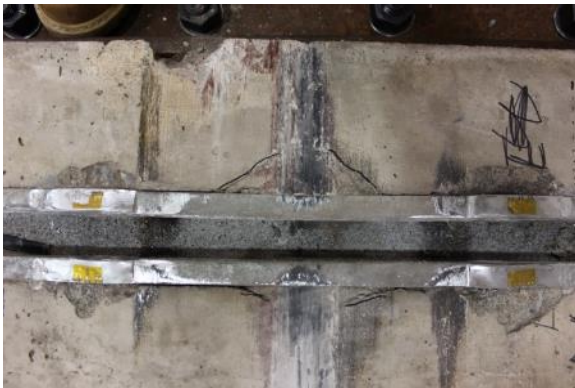
Cracks in the middle of a slab
