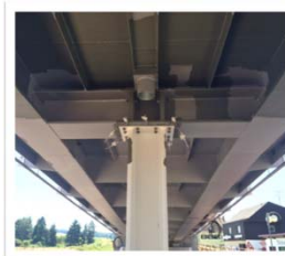
Steel flange connections
