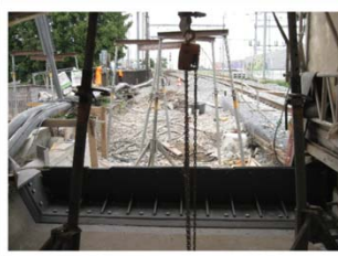
Broken rock walls
