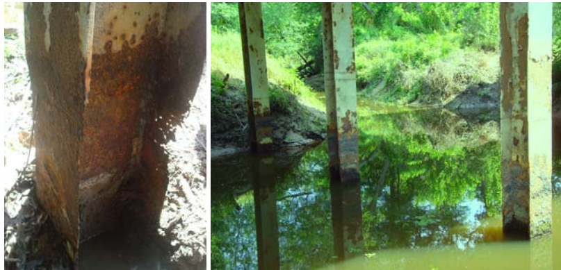
Figure 1: Deterioration of steel bridge piles
