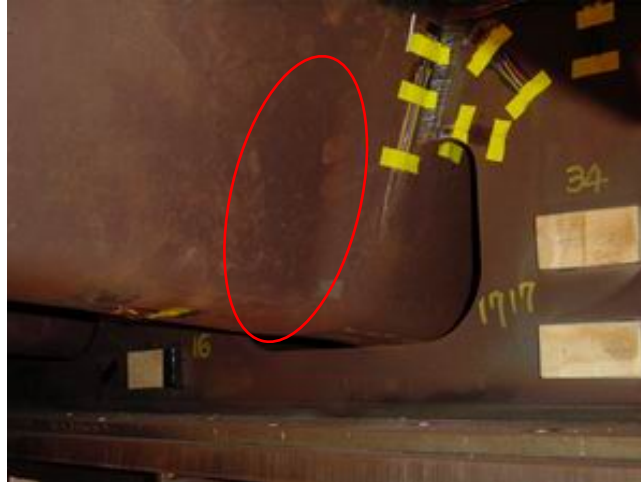
Figure 6: Closed up view of buckled rib wall of triple-rib Beam
