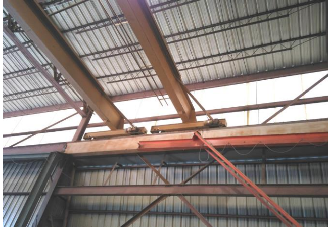
Figure 1: Two monorail crane bridge girders supported on top-flange of runway beam
