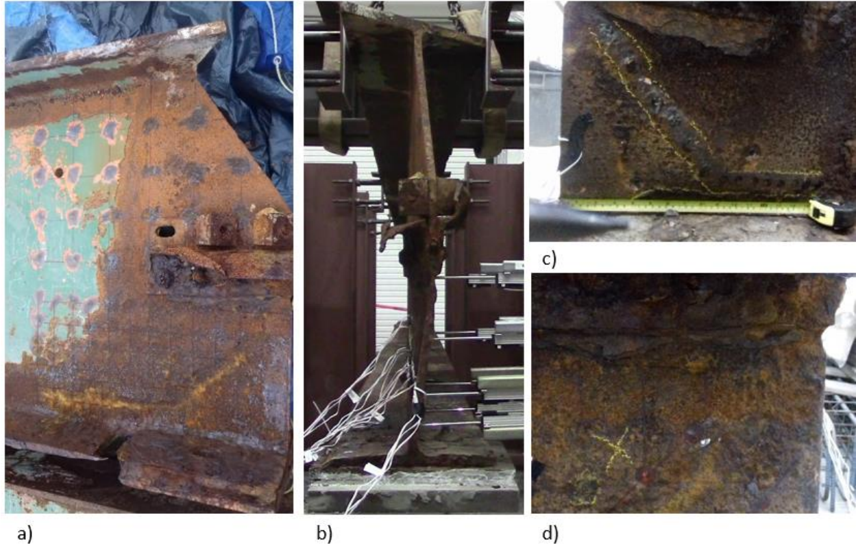
Figure 2: a) The corroded end of specimen 2 b) The maximum initial lateral displacement equals to 1.58'' c) The two areas with extensive section loss at second's specimen web d) A quarter inch diameter hole, located 4 inches below the steel angle sections.
