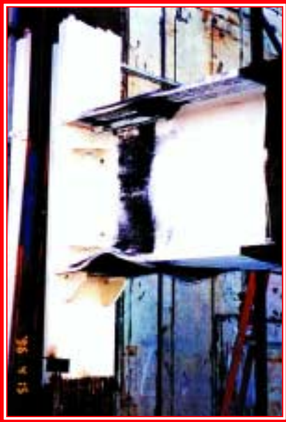
Figure 13: Hinging and buckling at -7 Delta yield for the W36x280 beam
