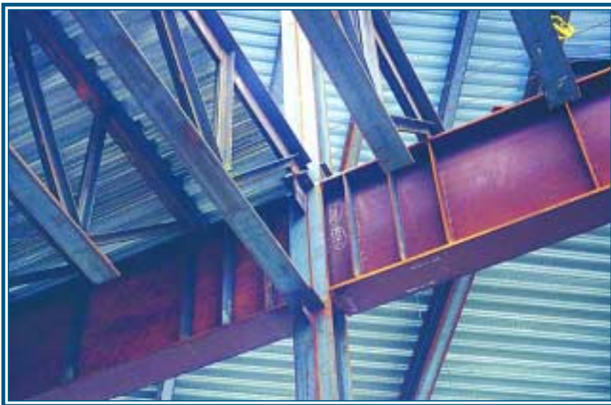
Shown on the opposite page is the roof beam to column connection. Pictured above is the steel joist connection at column and plate girder at column.
