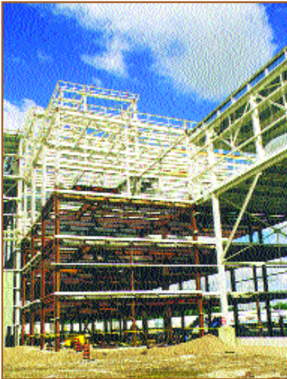
Recent work by Steel Plus members include such projects as the Southbend Riley High School in Southbend, IN (top) and a Chrysler plant in Windsor, Ontario (above).
