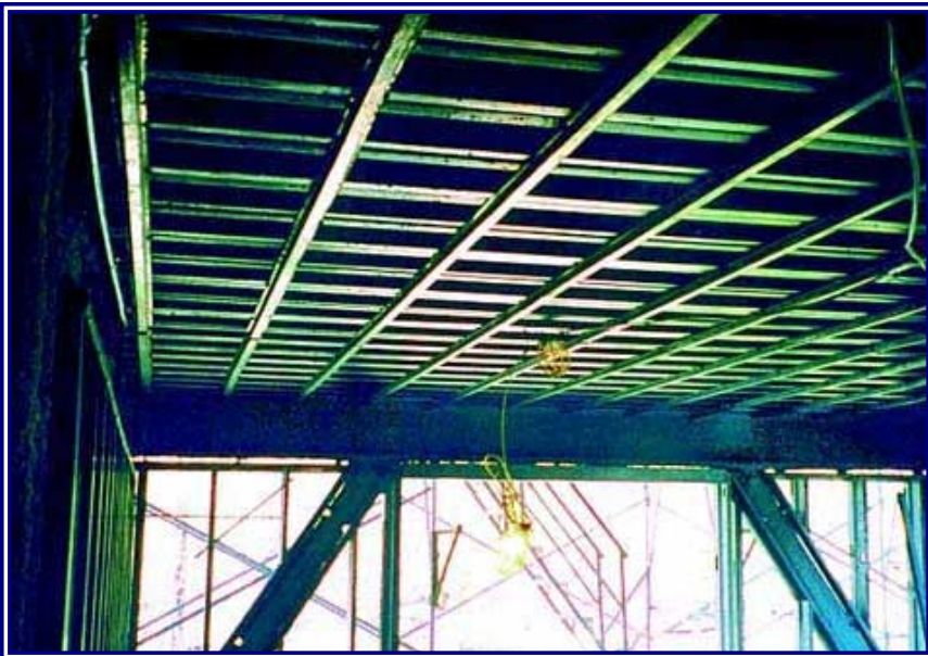
The underside of the composite floor deck is seen with furring channels applied for the gypsum wallboard ceiling. Beyond are the diagonal braces spread apart to accommodate the window opening.
