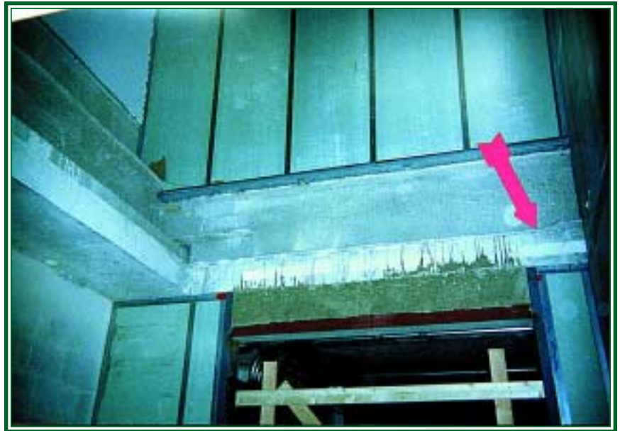
The new elevator shaft opening reveals the cross-section of the existing wideslab floor.
