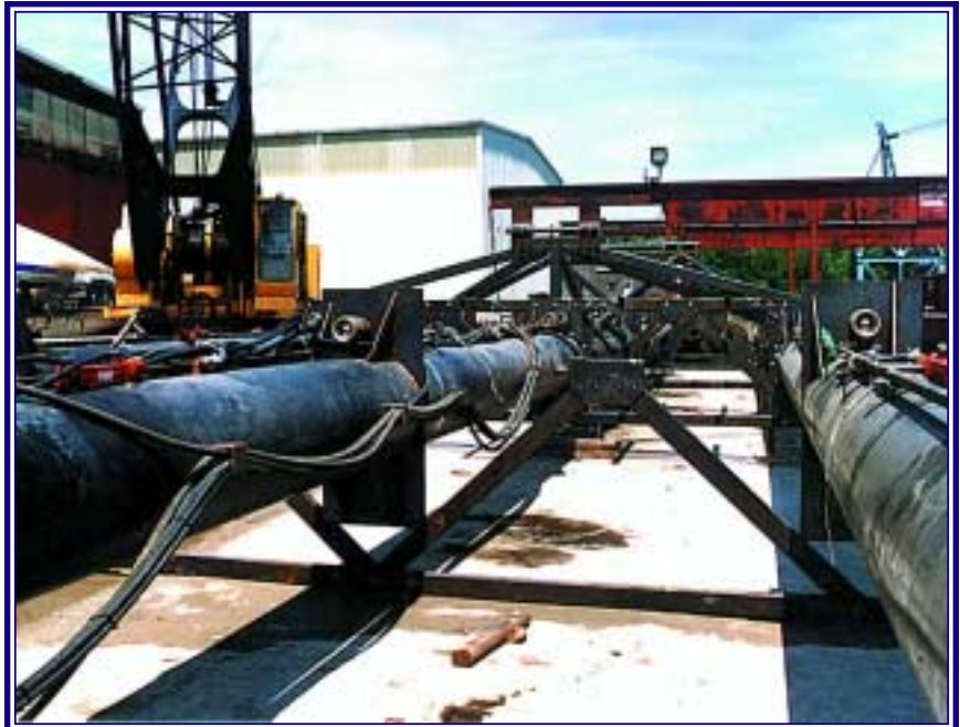
Shown above is the floating gimbal being assembled for transport to the Ohio River site. Visible are longitudinal pipes, transverse trusses and fuselage connections.
