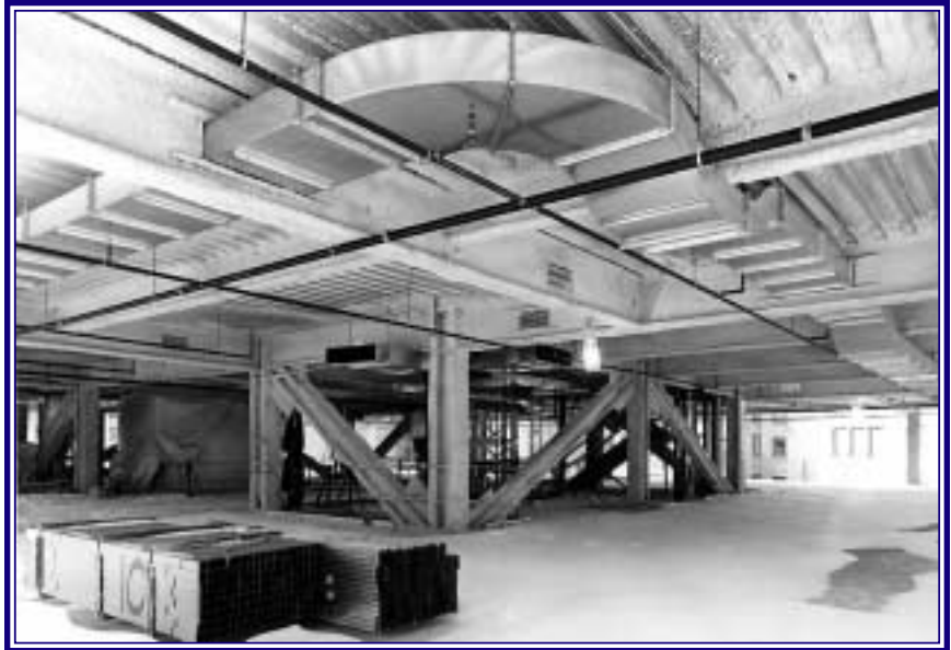
The layout of the core was designed to allow for diagonal members to be located in each direction on all four sides of the core.
