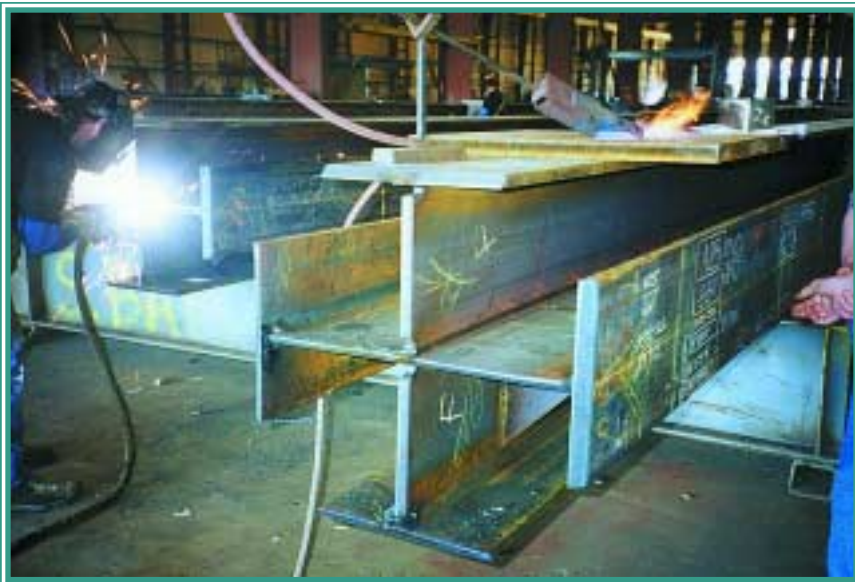
Pictured above and on the opposite page are the roof trusses and T-Y-K joints during fabrication and erection.
