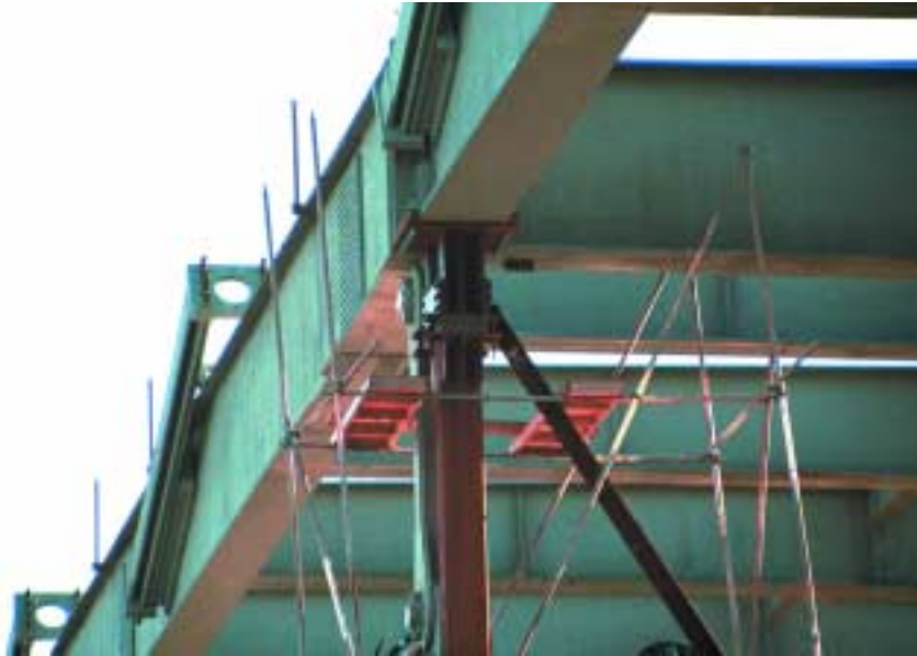
The construction photo above was taken during the positioning and leveling process of a girder on falsework, while the photo opposite shows work on the strands.
