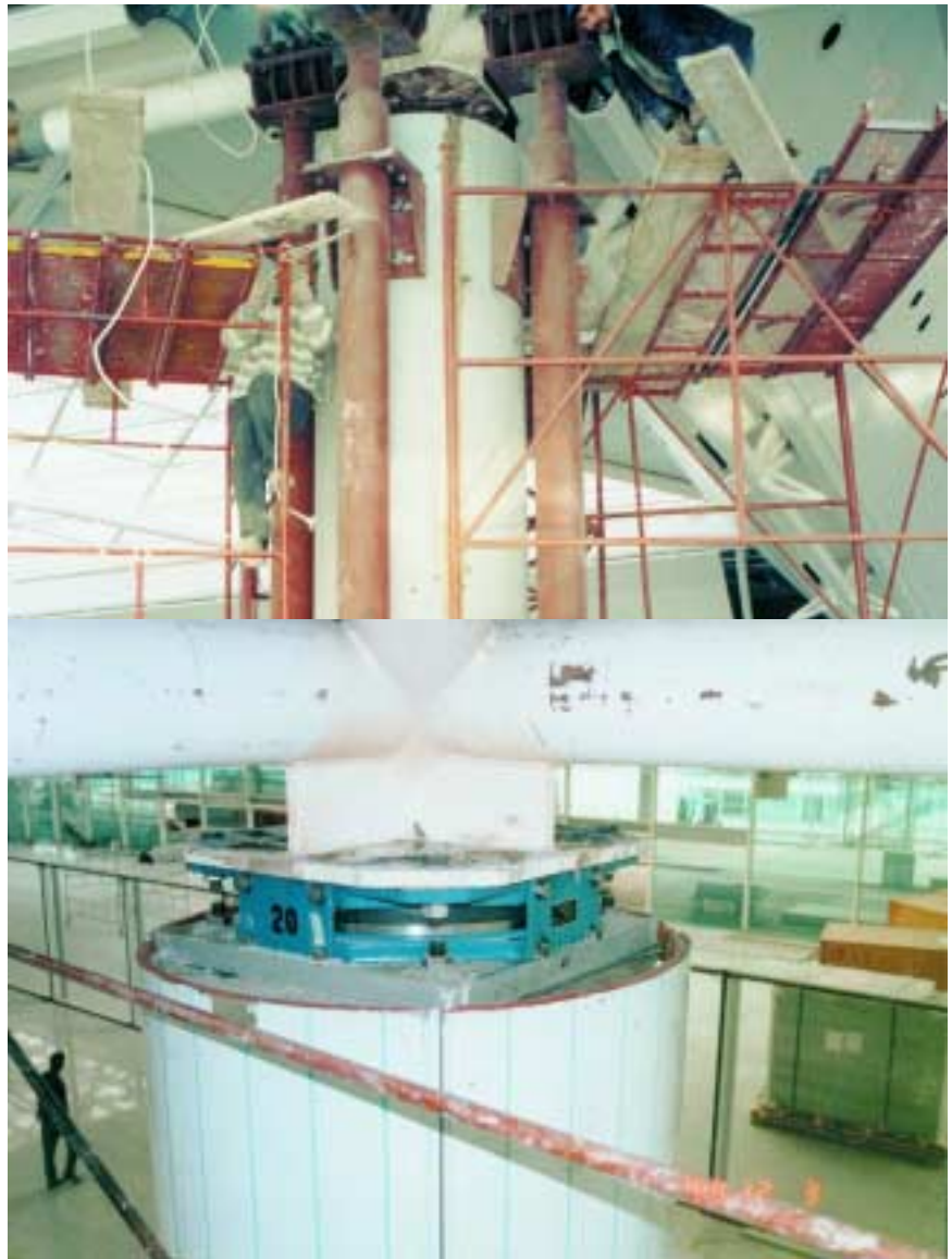
Top: Jacketed column with temporary bracket..
