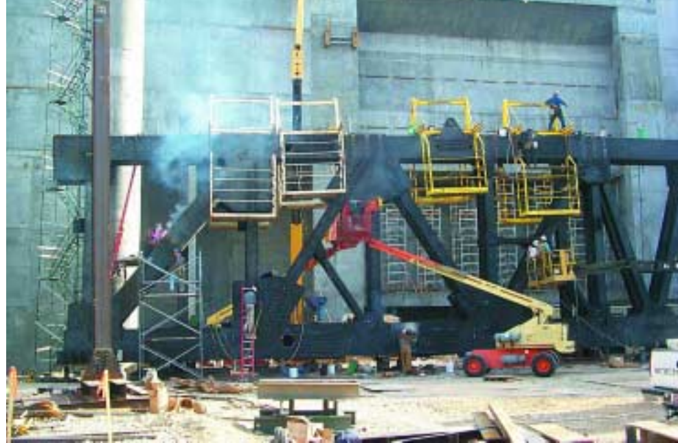
King truss—field welded splice of ASTM A709 30"x50" box - 2 1/4" plate compression diagonal.
