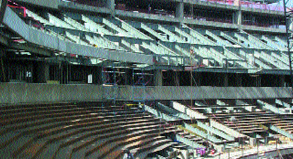
View of club (middle) and lower bowl framing and both levels of suites at north endzone.
