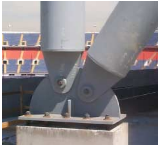
View of same typical pinned connection, as built (existing Mile High Stadium is in the background).
