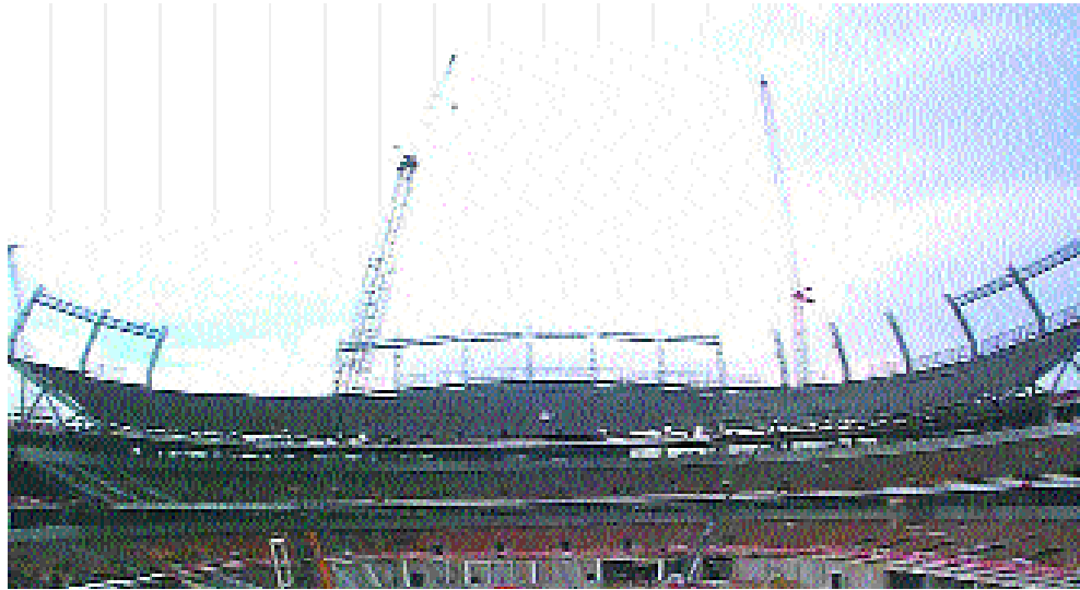
View of north (enclosed) endzone upper bowl, taken from south (open) endzone.
