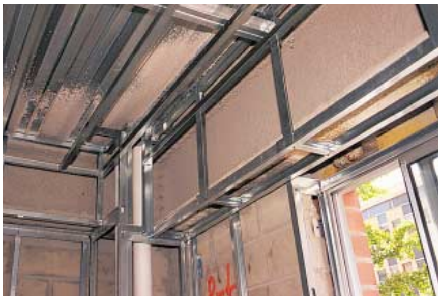
View of metal deck and fire-protected beams prior to gypsum board installation.
