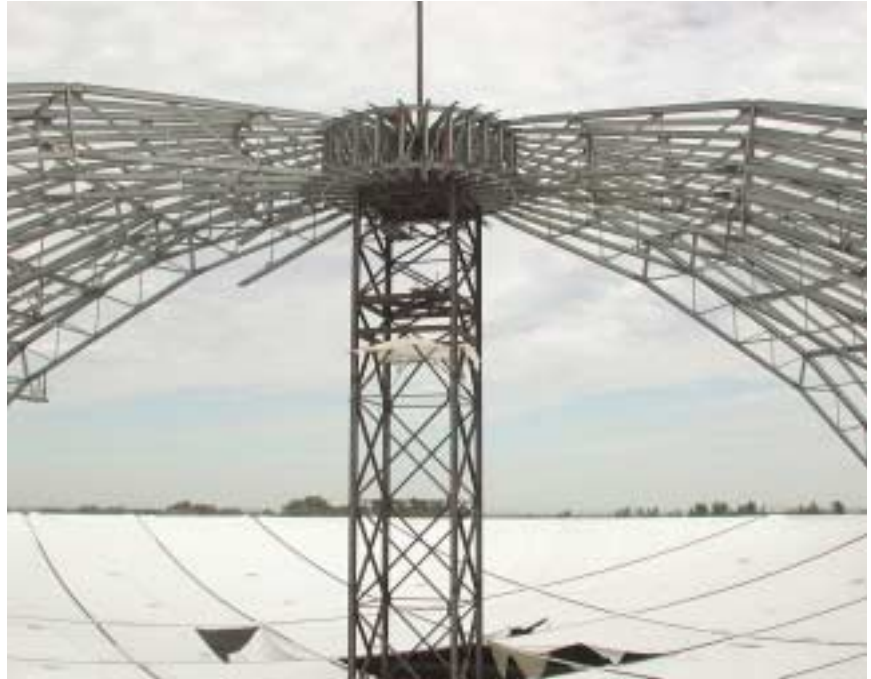
View from the existing concrete ring beam showing the balanced erection of the partially erected dome. (The existing roof fabric is pierced by the shoring tower).
