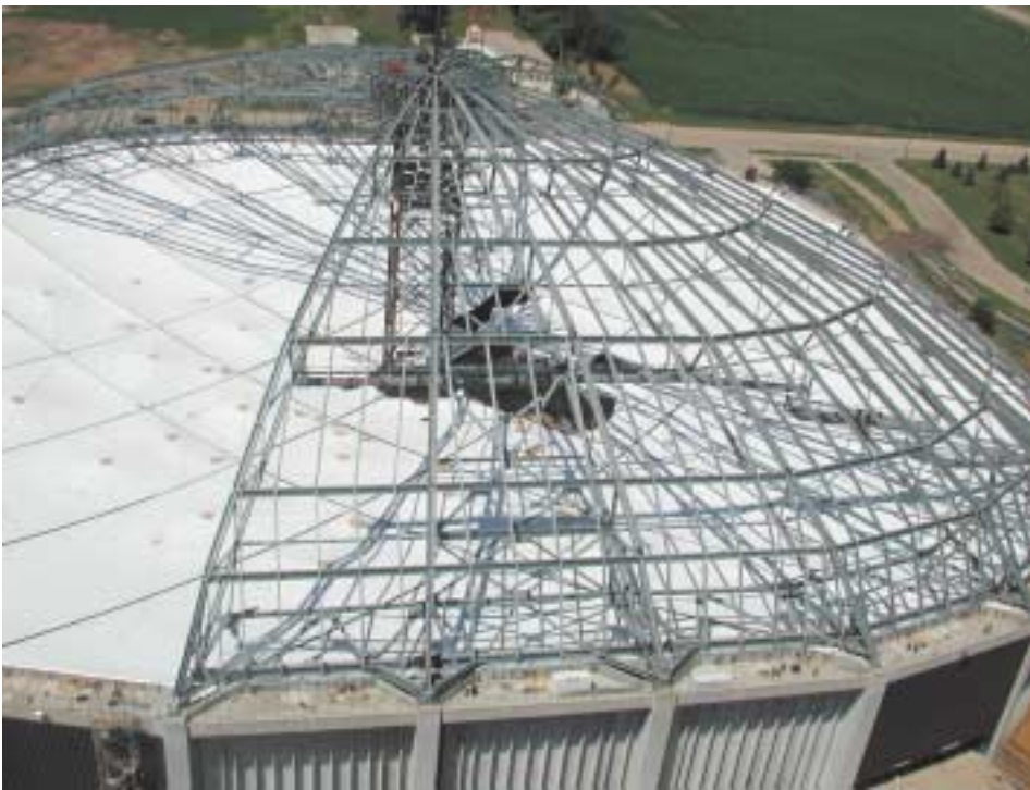
Aerial view of partially completed internally resolved dome structure taken from 300' boom erection crane.
