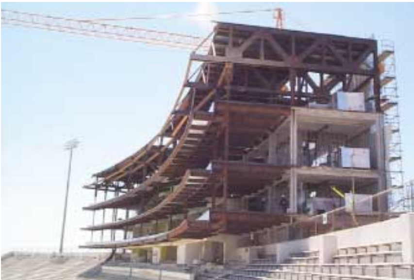
The truss bents are clearly visible in this construction photo of the Bear Heights level looking southwest.
