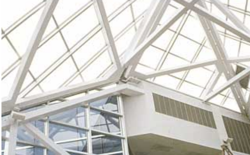
Detail of atrium panel framing and joints including one of the support seats.
