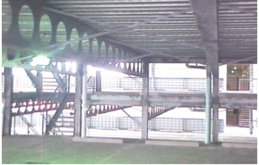
Interior view of completed garage. Note the x-bridging, used to stabilize the long-span steel members during erection.
