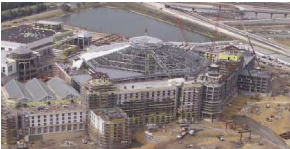
Opposite page: The Everglades Atrium features an acre of glazed roof. Four Pratt trusses, 11' deep, form the primary structure.
