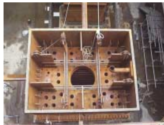
View of super-column shell. At the base, the super-columns are 2.4 m by 3.0 m (approximately 8' by 10').
