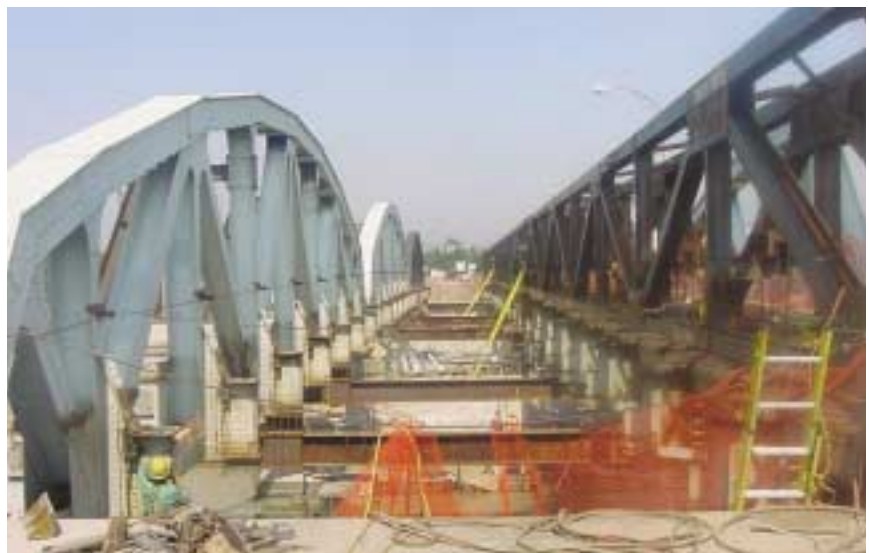
The old deck and floor beam were dismantled and replaced. The existing trusses, moved outwards from their original locations, support the sidewalks for the reconfigured bridge.
