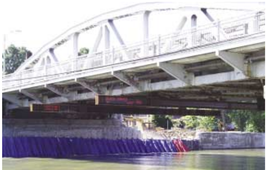
Temporary beams, attached to the bottom chords of the temporary trusses, supported the existing trusses as they were disconnected from the bridge structure and slid outward.
