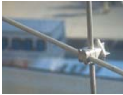
Cable net wall for the AOL Time Warner Building in New York with stainless cast steel corner patch plates and cable clamps
