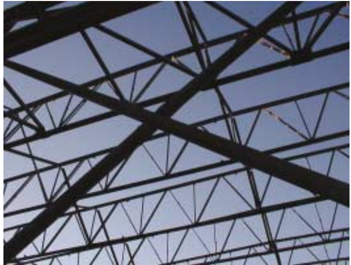
View of tubular X-brace and roof framing during construction of the natatorium.
