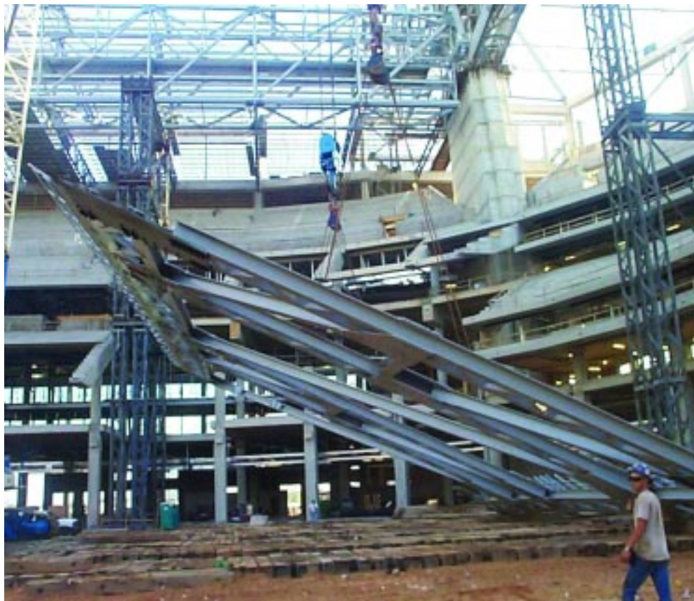
A 400-ton crane and a 650-ton crane perform a tandem lift of a fabricated side section of the east supertruss. The scoreboard box truss (still supported on erection towers) can be seen framing into the left side of the concrete supercolumn.
