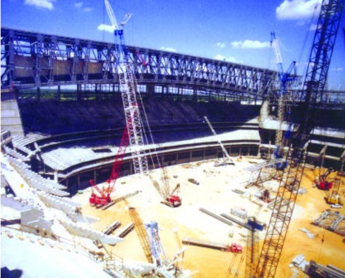
The erection towers have been removed from beneath the west supertruss. The lacing of the truss chords and vertical web members are visible in this picture. The first fabric panels have been installed on the left end of the main truss span.
