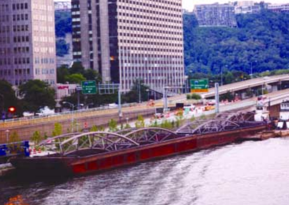
Trusses being delivered to Pittsburgh on barges. These trusses were then trucked across the city to the job site.
