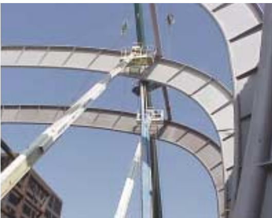
Seventeen curved, steel-bent beam-columns or "ribs" support the roof structure. The ribs were erected in two pieces with a bolted and welded splice connection approximately 60' above grade
