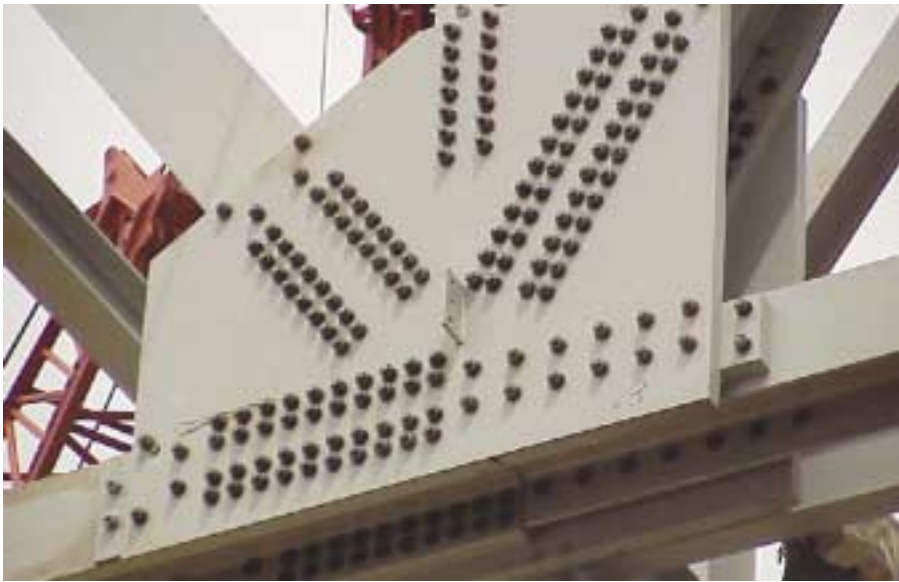
Some of the gusset plates in the box truss are more than 3" thick
