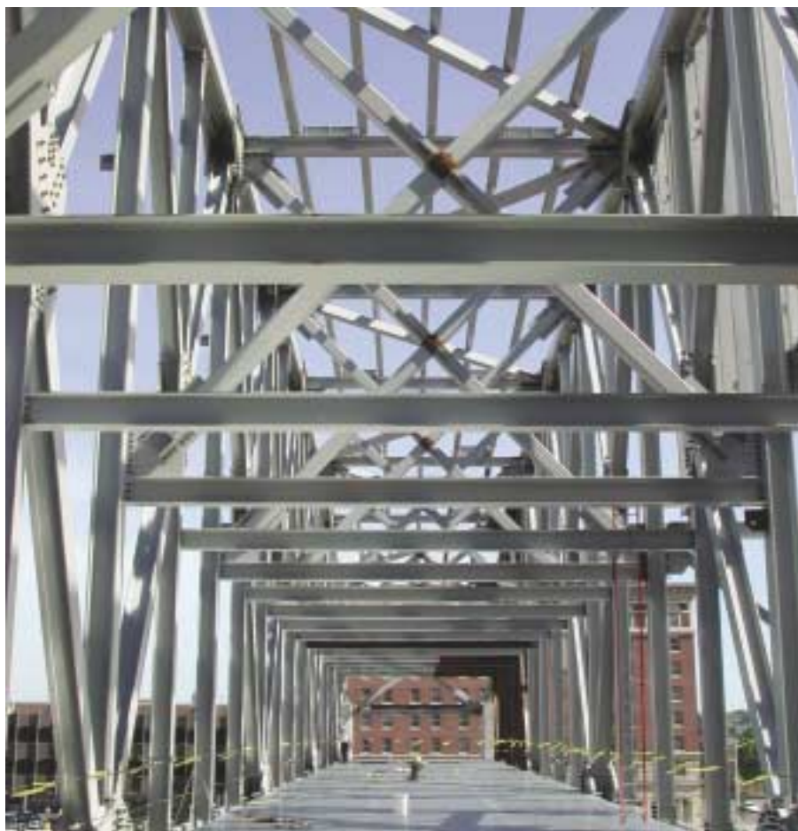
Longitudinal view through one of the two steel box trusses supporting the roof structure.
