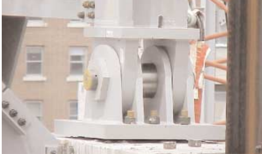
The box trusses connect to each concrete pier with a pin assembly connection.
