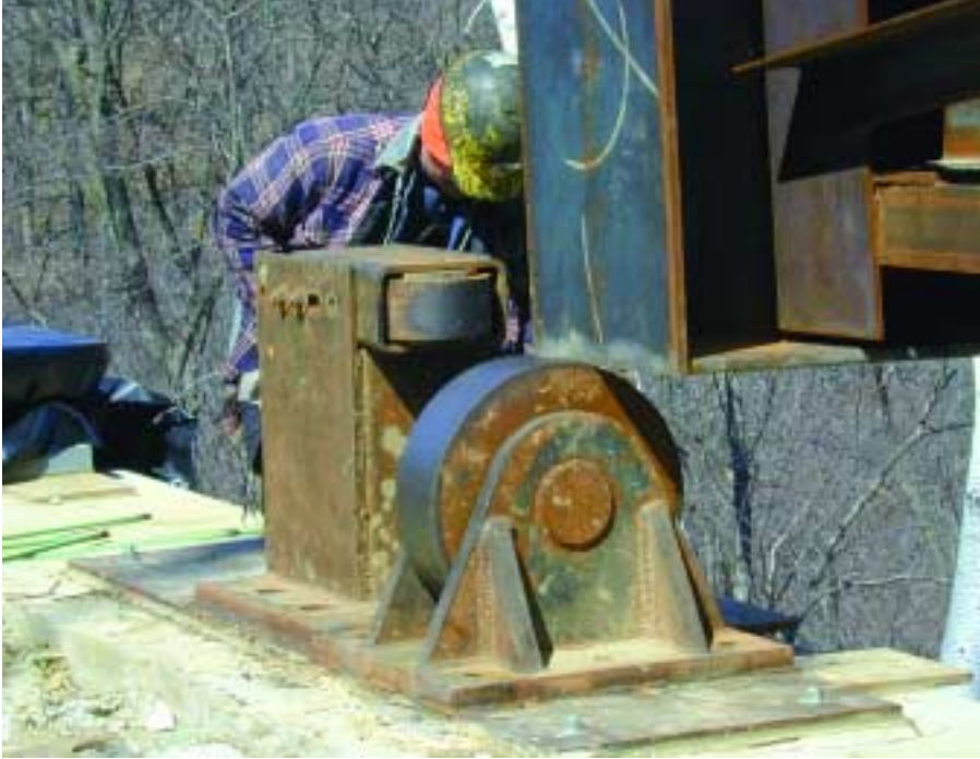
Vertical bearing rollers supported the mass of each girder on its bottom flange, and horizontal guide rollers provided alignment control at each bent.
