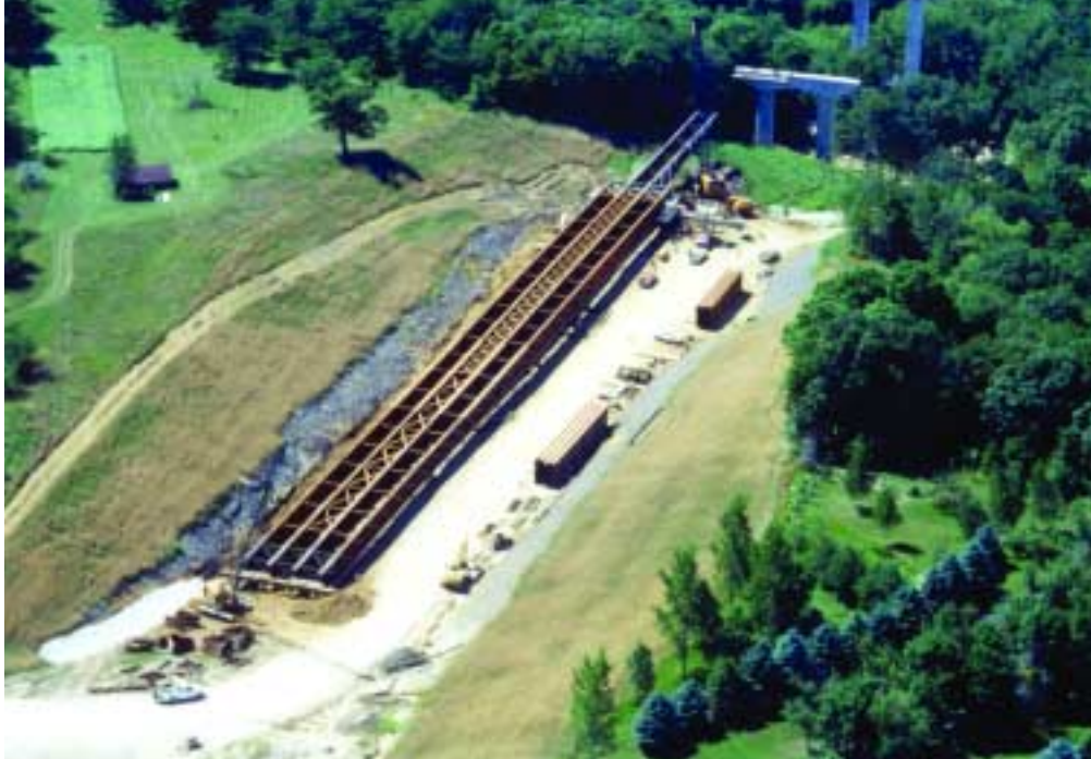
Above: A launching pit excavated behind the east end of the span was approximately 200 m long by 36 m wide by 6 m deep (660' by 120' by 20').
