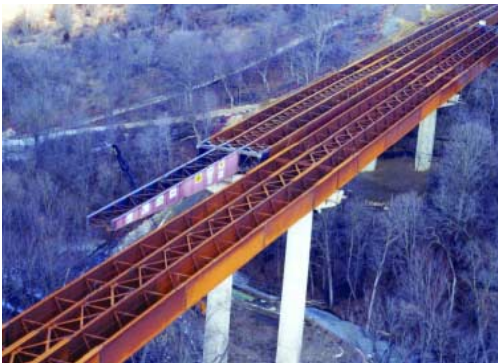
Below: The tapered "launching nose" bolted to the girder allowed the deflected cantilever to "catch" each bridge pier as the launch progressed.
