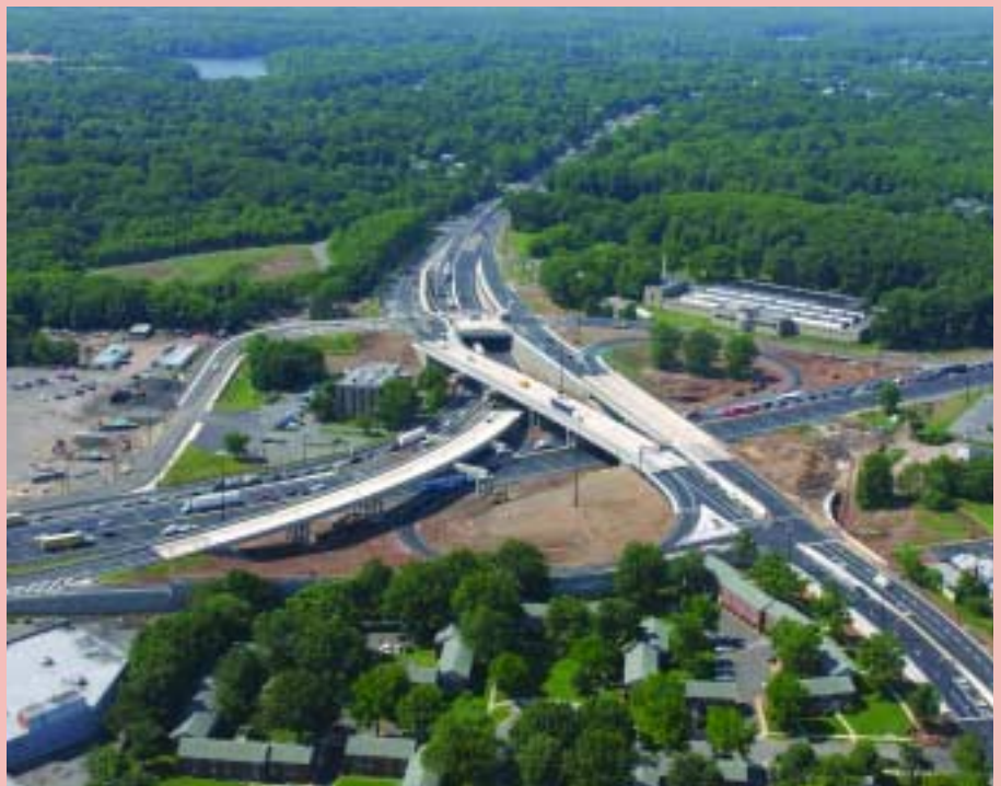
New Jersey DOT interchange project linking Routes 1, 130, and 171 made extensive use of electronic document approval to meet 18-month timeframe.
