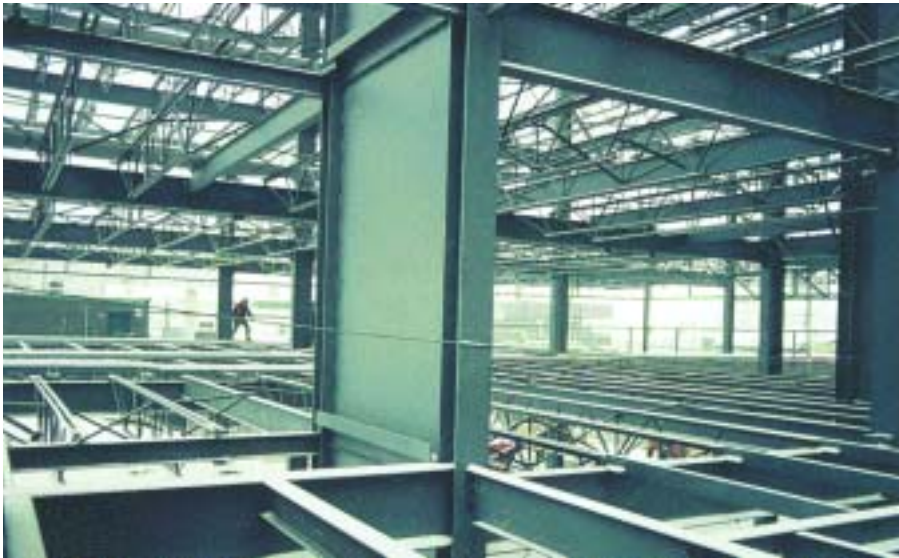
Planar SPSW (Canam HQ). See the September 2001 issue of MSC at www.modernsteel.com .
