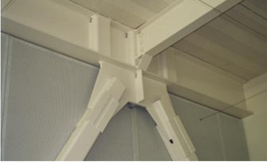
For tension, the exposed braces are reinforced by four angles mounted over the corners of the square HSS brace. These angles provide additional area to prevent a weak section where the brace is slotted to fit over the gusset plate.
