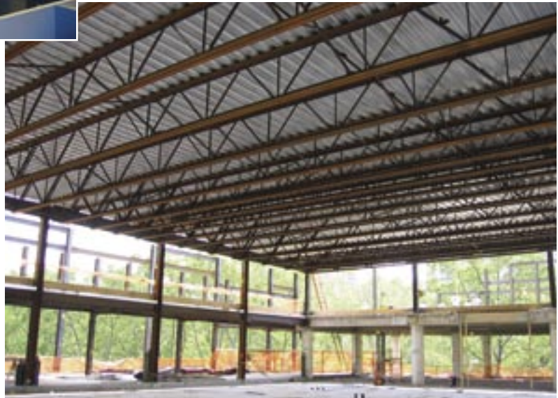
The new Emergency Operations Center (shown nearly completed, top) required a 70-ft by 100-ft open space.
