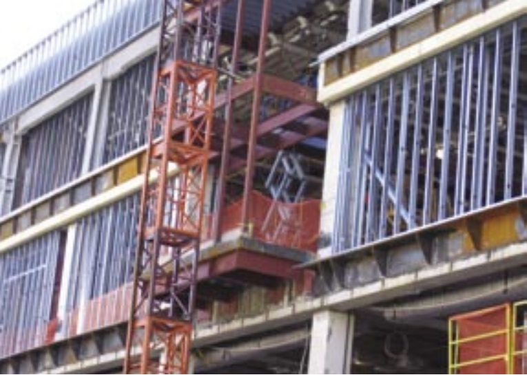
Shelf angles to support the new facade were attached to the existing concrete using Hilti anchors.
