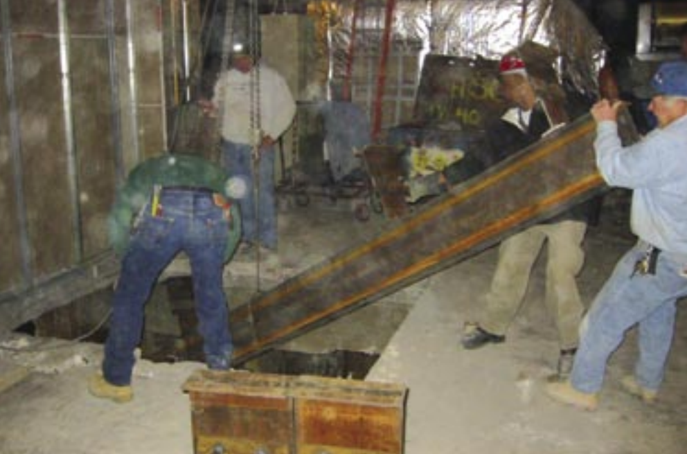
All construction materials were brought to the top of the building using the existing freight elevators.
